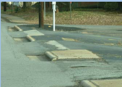
Sidewalk and curb cuts on W. Main in front of the Post Office
