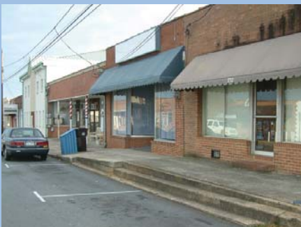
Grade issues on E. Main Street
