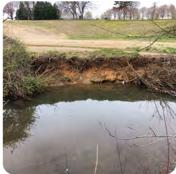
PHOTO: Heavy streambank erosion along Richland Creek within Blair Park Golf Course in High Point, March 2021
