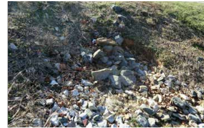
Figure 17: Clogged Culvert at Townbranch Rd
