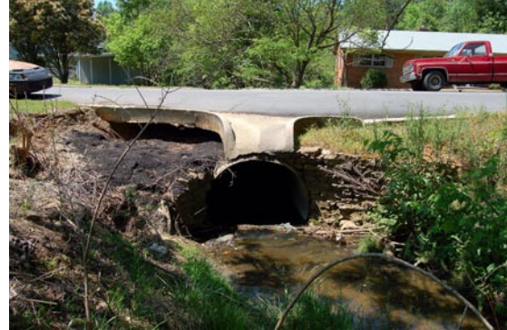
Figure 2: Failing Stormwater Culvert in Little Alamance Watershed
