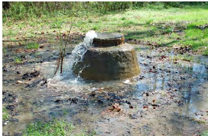
Figure 73: Sewer Overflow in Eden
