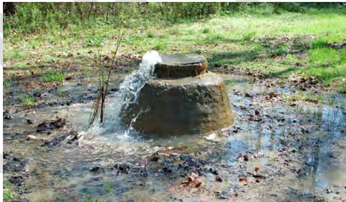
Figure 31: Sewer Overflow in Eden
