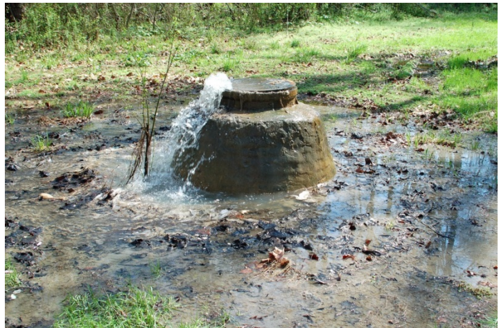
Figure 40: Sewer Overflow in Eden
