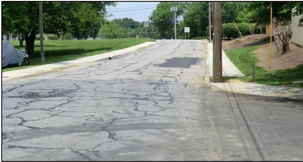
Figure 1: Pavement Conditions on Washington Avenue Looking North from Habitat Place
