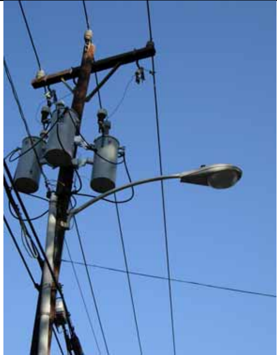
NEMA Standard of Cobra (Lebanon Ave.)
