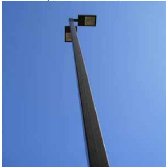
Small box 2-head (parking lot off Lebanon Ave)
